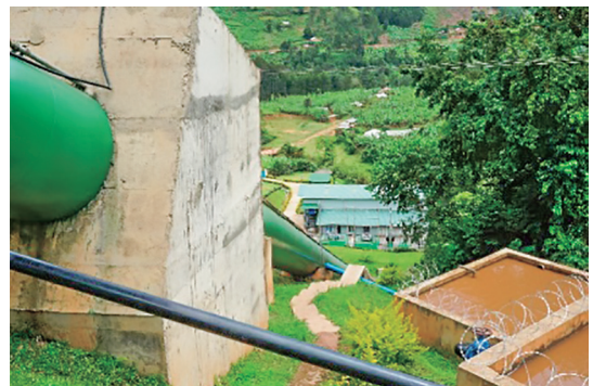
the hydroelectric generating station at Muvumbe
